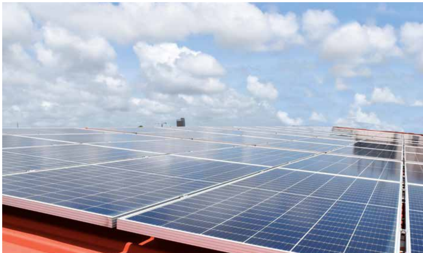
Solar panel at SDF Head Office Roof.
